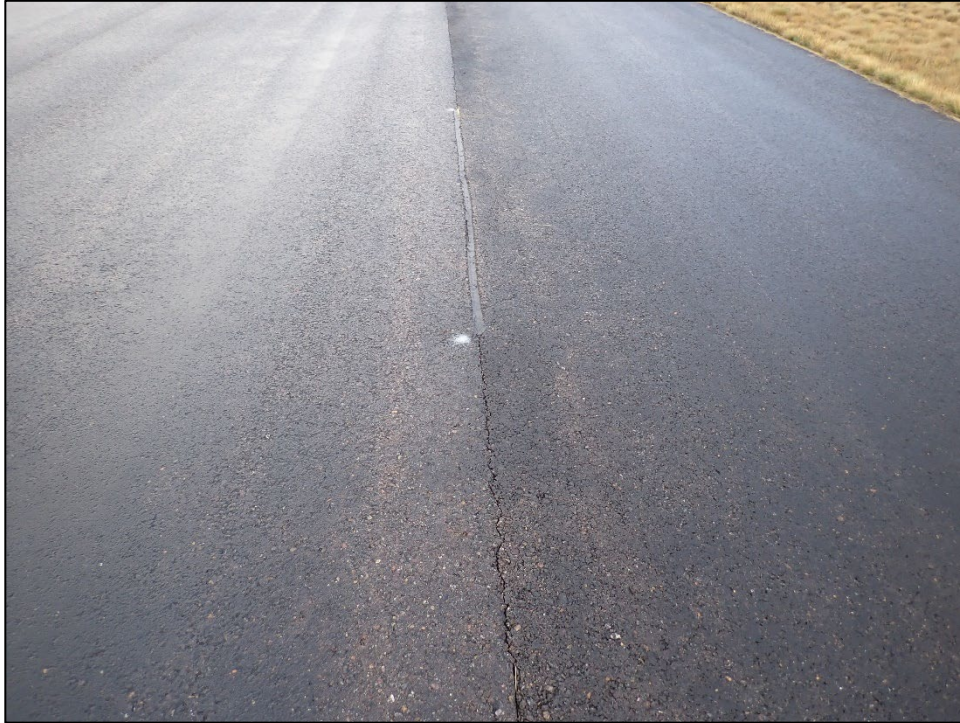
RW12-11-24: L&T Cracking
