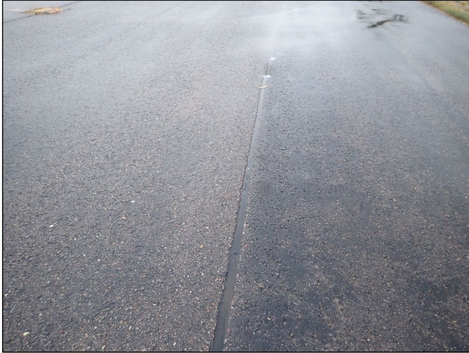
AP-11-03: L&T Cracking
