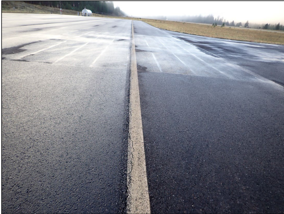
TW-11-02: L&T Cracking
